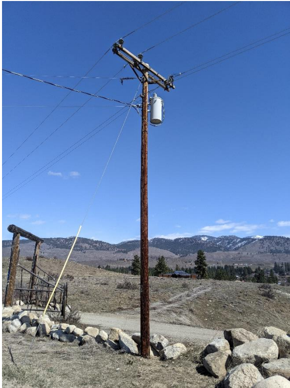
PRIMARY POLE WITH OVERHEAD TRANSFORMER
