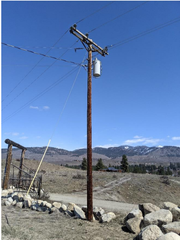
PRIMARY POLE WITH OVERHEAD TRANSFORMER
